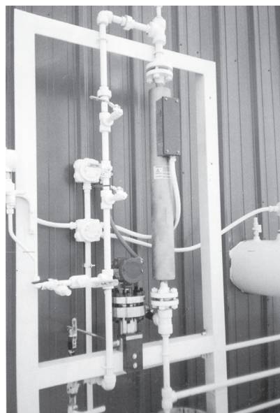
Typical installation. Note how the transducer is rigidly clamped, isolation valves are provided for easy maintenance.
